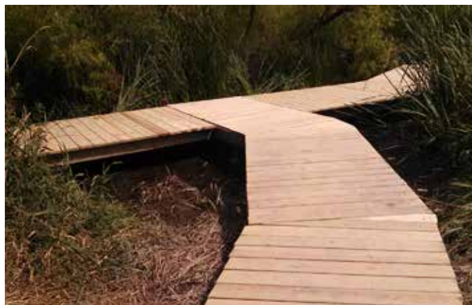
The boardwalk and belly boards at the north end of the North Unit were suffering serious frost heave before Operation Fresh Start's repair work. Photo by Jan Axelson
