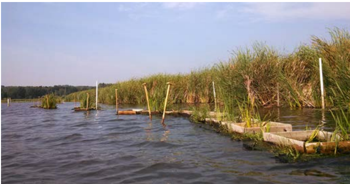
The floating bog interceptors (FBIs) are helping to prevent shoreline erosion at Cherokee Lake. Photo by Jan Axelson.
